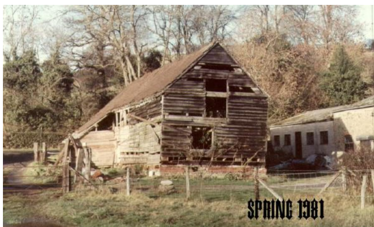
The barn in 1981 before work began to dismantle it and move it to Yarpole
